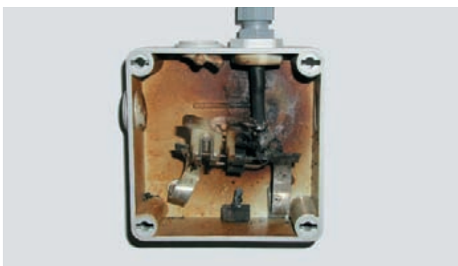
Module box after lightning strike
